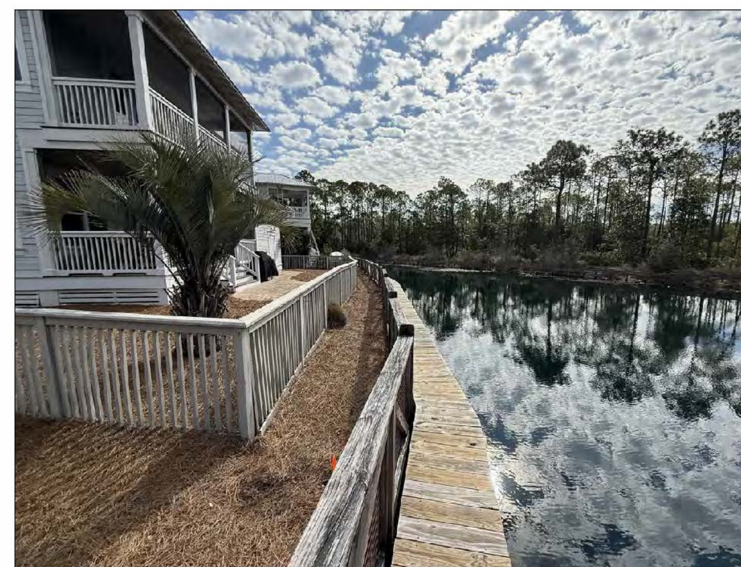
VEGETATION ENCROACHMENT ON LOT 89
