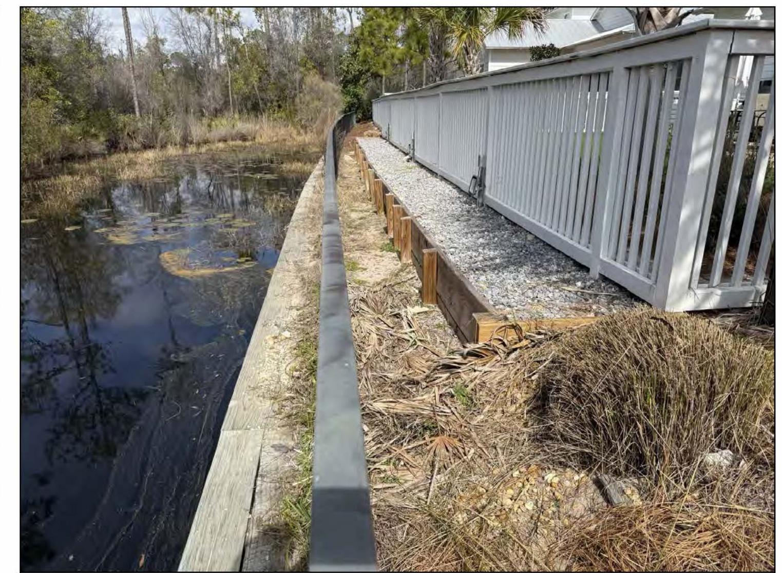
FILL/WALL ENCROACHMENT ON LOT 269
