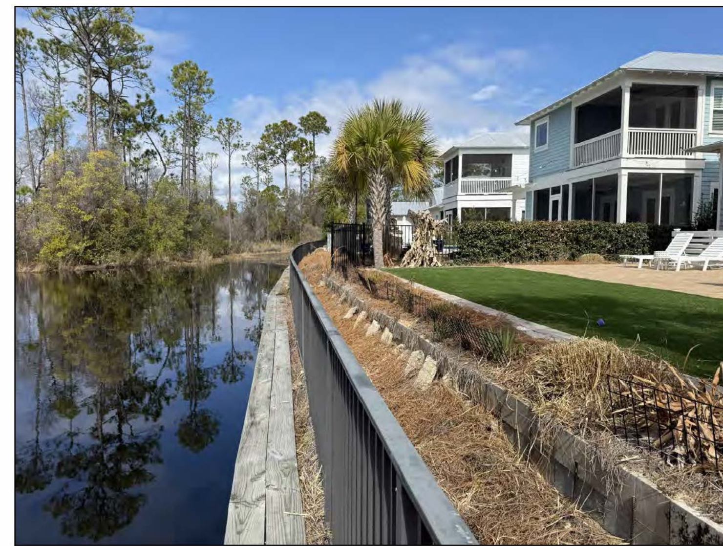
FILL/WALL ENCROACHMENT ON LOT 267
