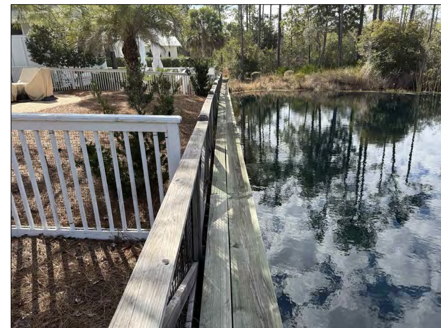
FENCE ENCROACHMENT BETWEEN LOTS 131 & 132
