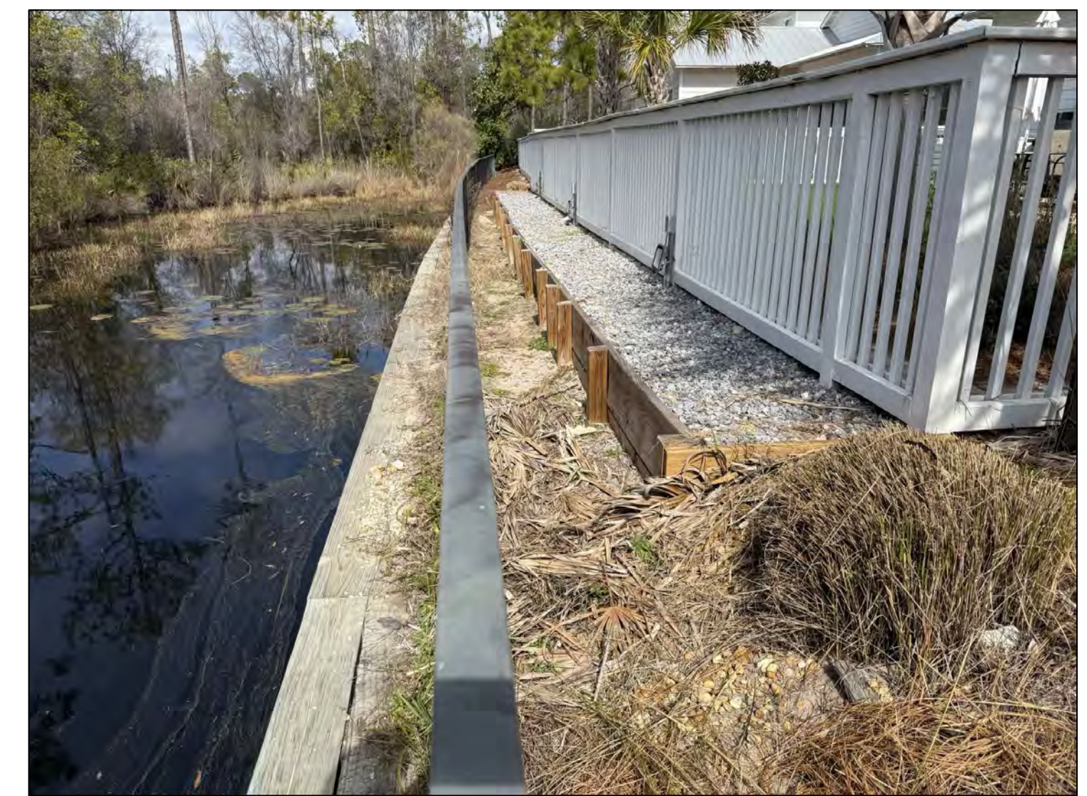
FILL/WALL ENCROACHMENT ON LOT 269
