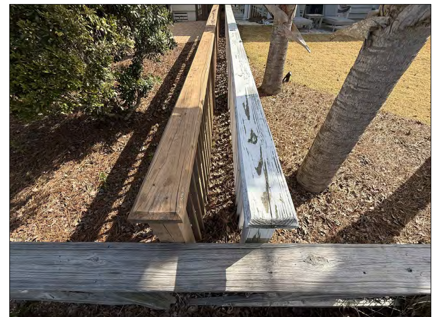
FENCE ENCROACHMENT BETWEEN LOTS 132 & 133
