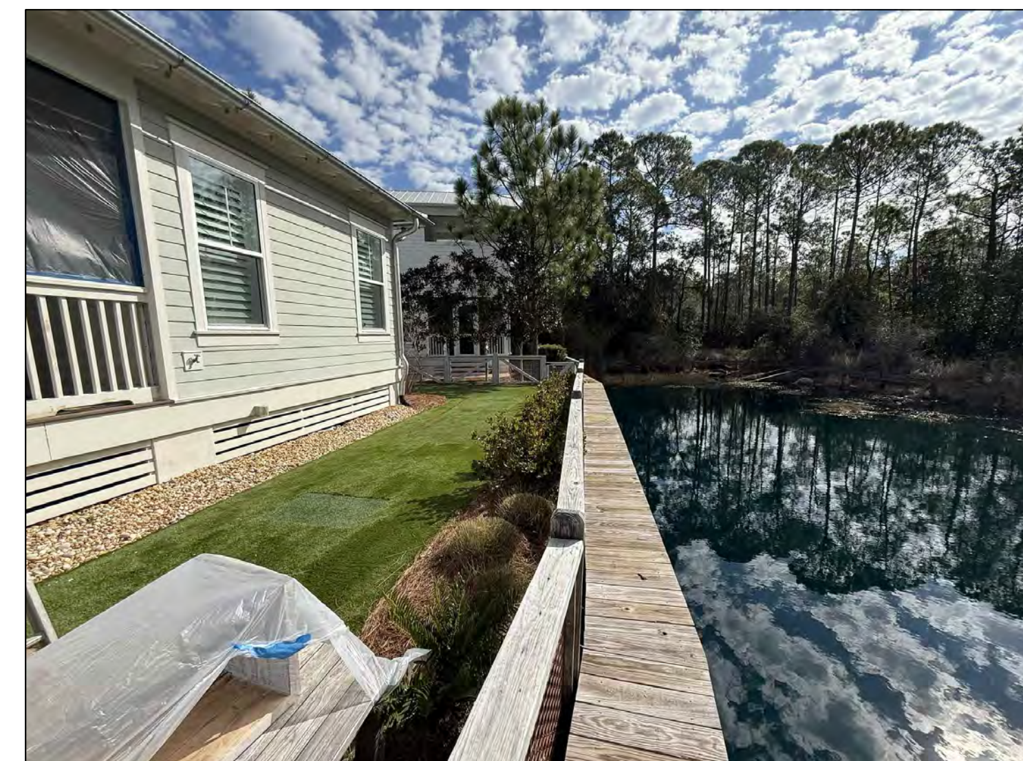
VEGETATION ENCROACHMENT ON LOT 90
