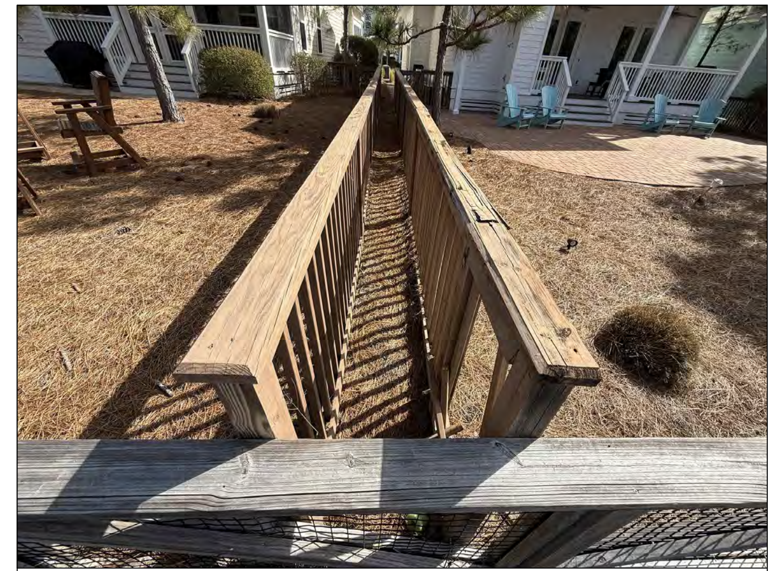
FENCE ENCROACHMENT BETWEEN LOTS 134 & 135
