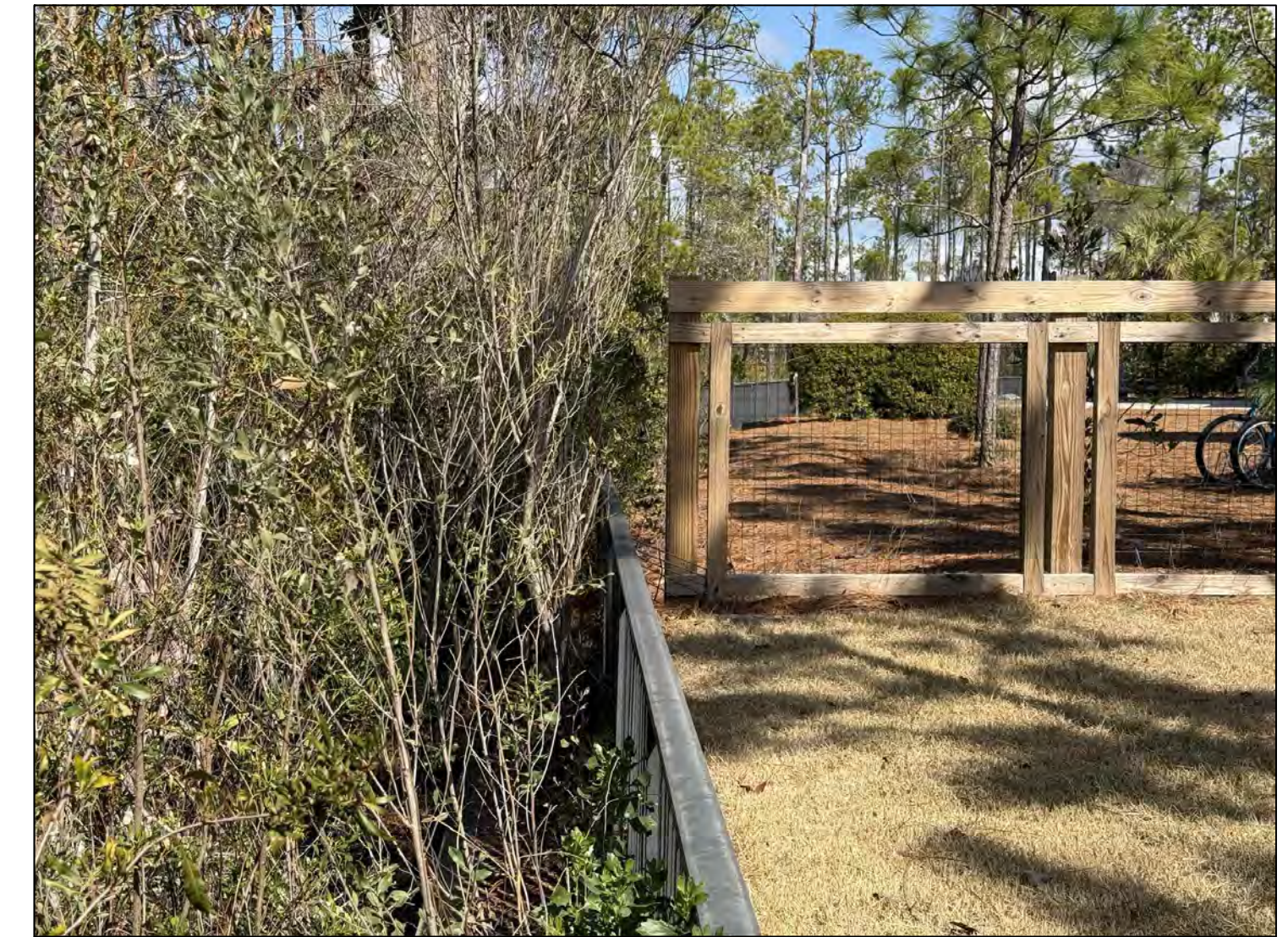
FENCE ENCROACHMENT BETWEEN LOTS 257 & 258
