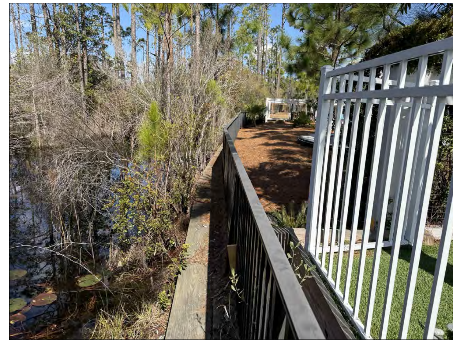
FENCE /WALL ENCROACHMENT ON LOT 254
