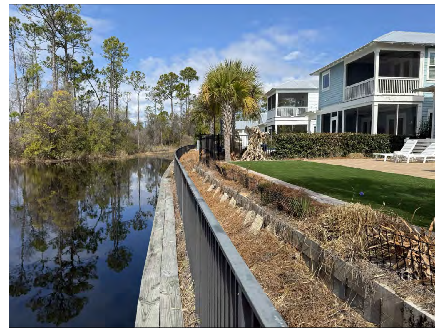
FILL/WALL ENCROACHMENT ON LOT 267
