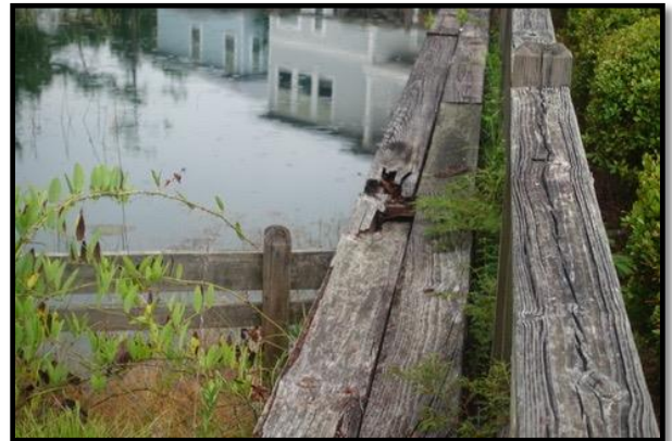
Figure 2 – Wood Cap Rot
